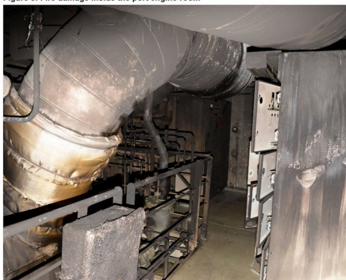
Figure 8: Fire damage inside the port engine room
