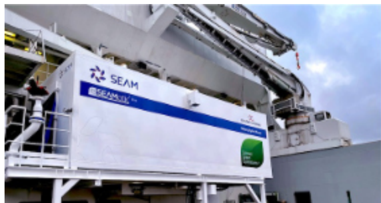
Part of SEAM's eSEAMatic blue hybrid installation on a Solstad Offshore vessel.
