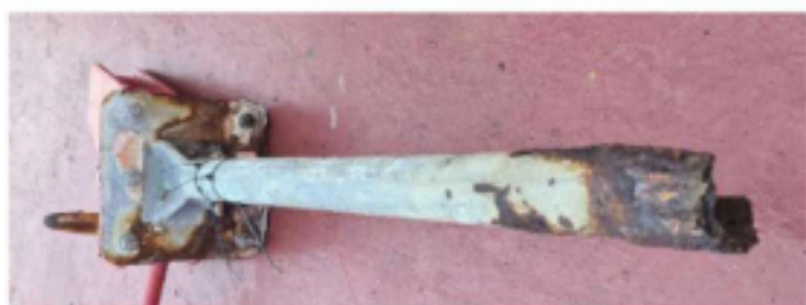
Figure 1: Photo of the rescue boat release hook support structure taken after the incident, showing significant deterioration of the post.
